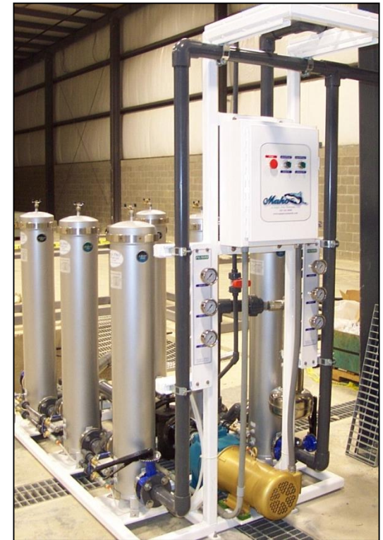
Twin Filtration Array
